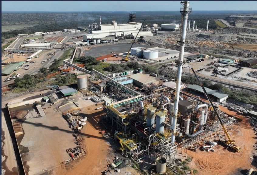
Acid Plant #5: 900 tpd
