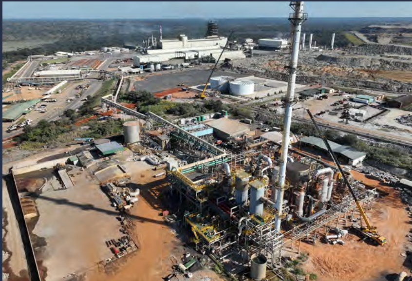
Acid Plant #5: 900 tpd
