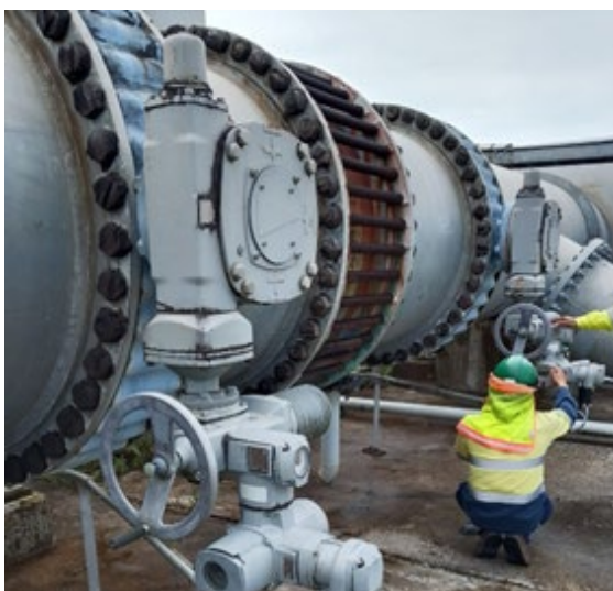
Process – Water pump valve change
