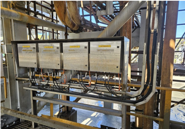
Refurbished flotation pump valve control cabinets
