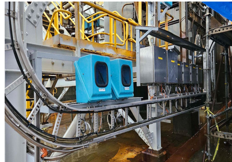
Renewed cleaner flotation cable trays and instrument station covers
